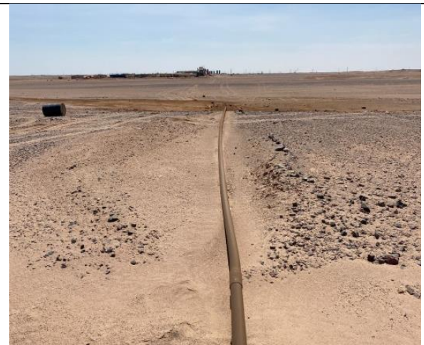
Figure 92: Petroleum Pipes (Site 8)
