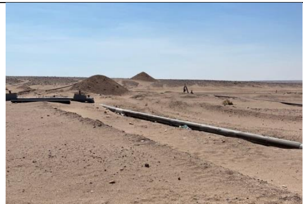
Figure 90: Petroleum Pipelines (Site 6)
