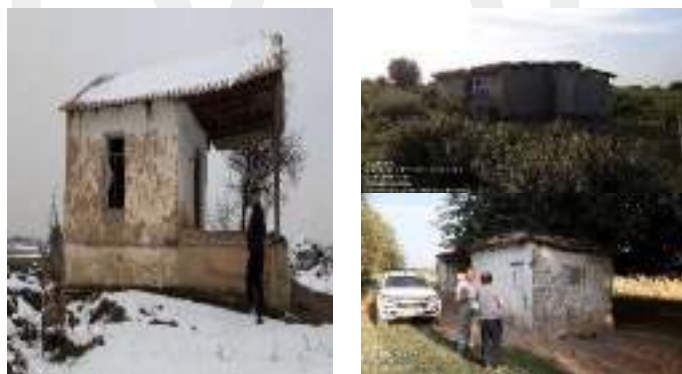
Figure 7-12 Seasonal dwelling for crop farm stay overs (left), seasonal dwelling (bottom right) and nearby crop farm shed (top right)
