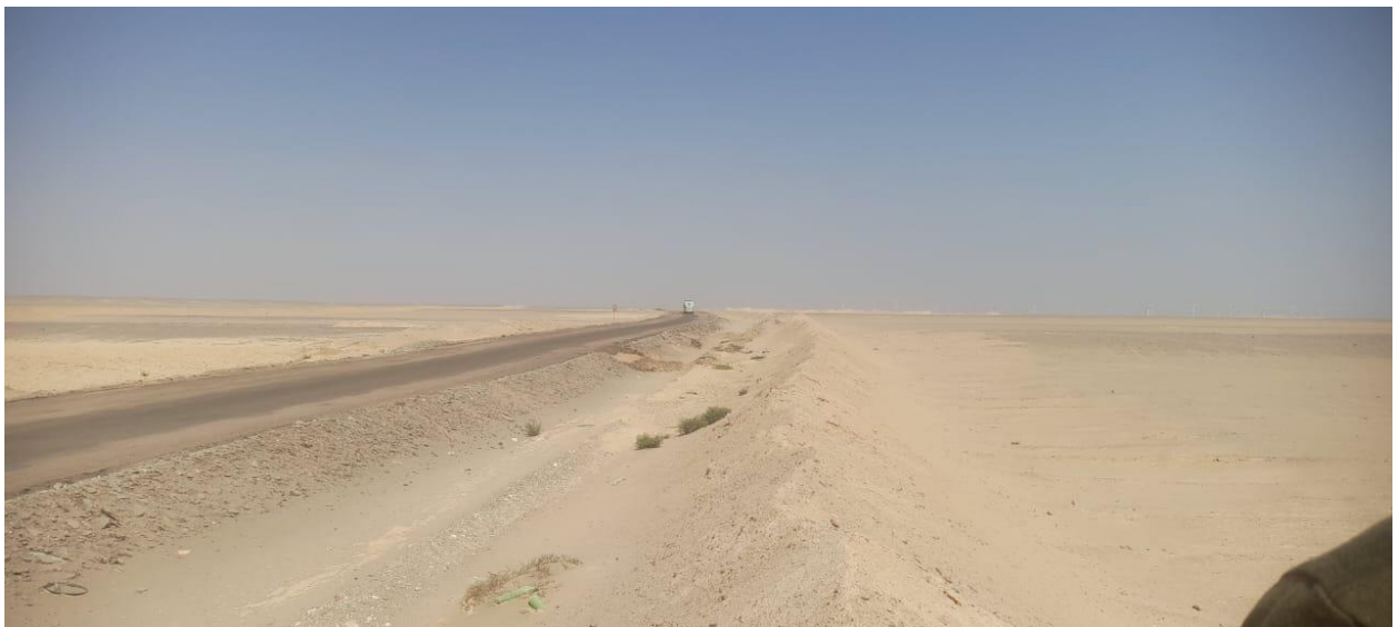
Photo 2.8: Road with high rubble beside it, and cutting in road as a result of torrential rains
