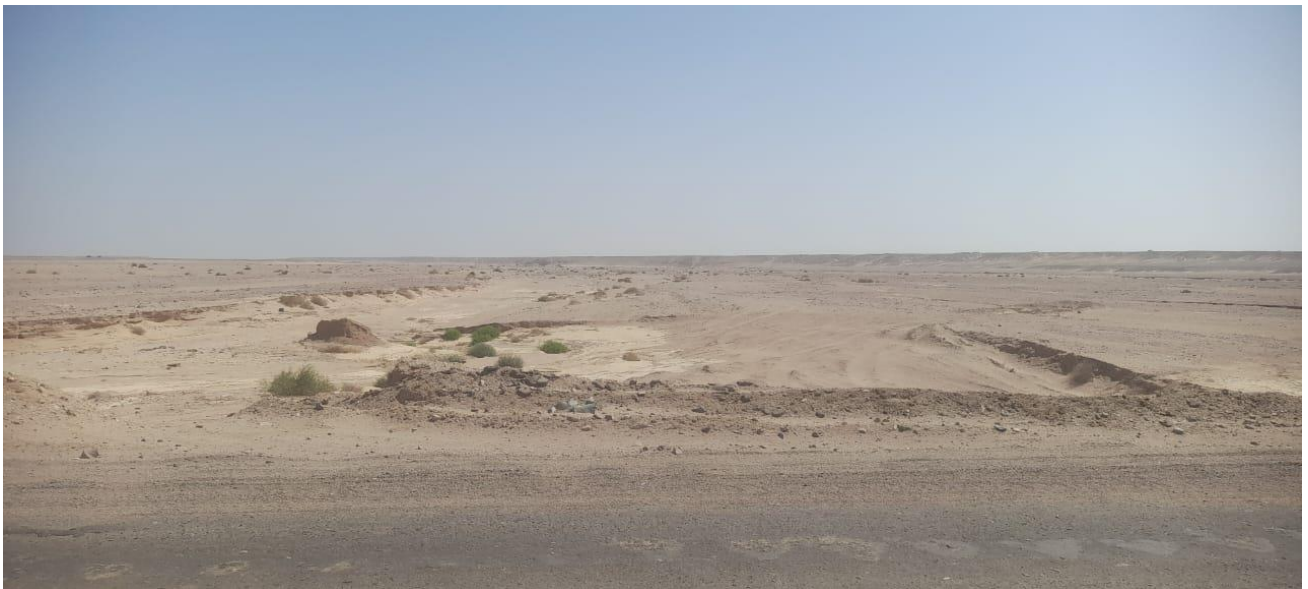
Photo 2.4: One of the Wadis after attacking the road inside the site, and the cut that occurred in the road as a result of attacking the valley
