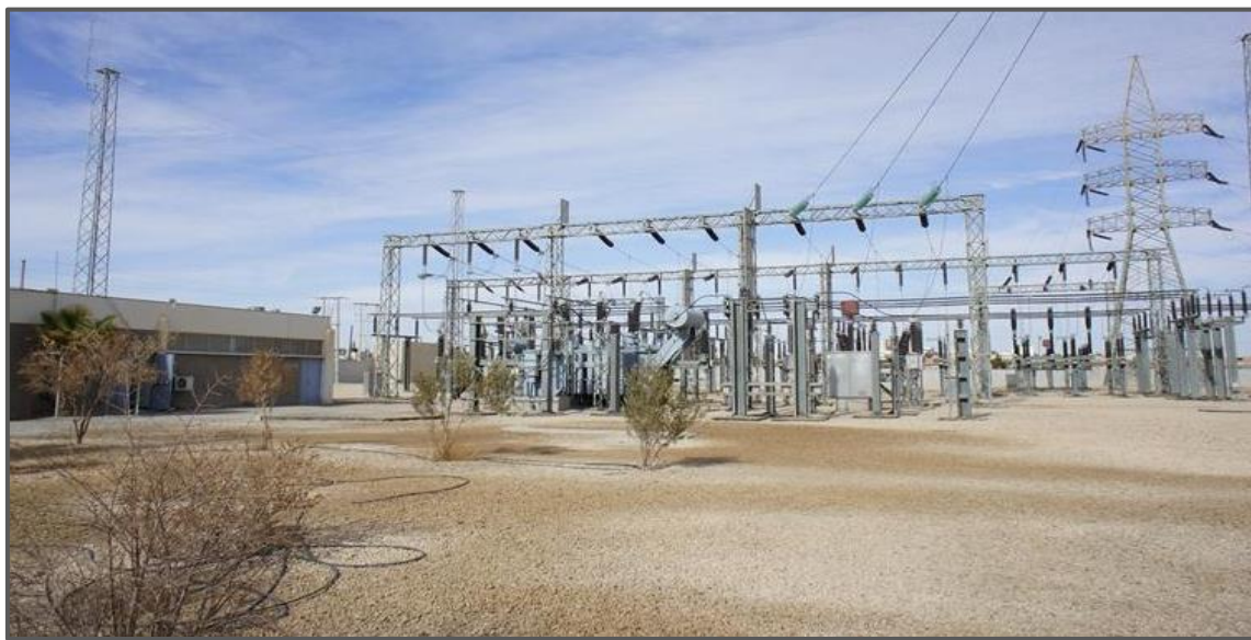
Figure 21: Typical 33/220kV Substation
